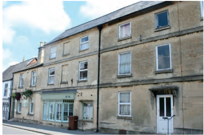
Fig 17.3: The effect of the loss of traditional fenestration can transform simple elegance into plain ugliness.
