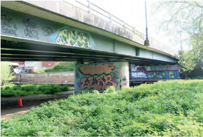
Fig 10.8: The underneath of the bridge has been put to good use as an informal gallery for community street art.
